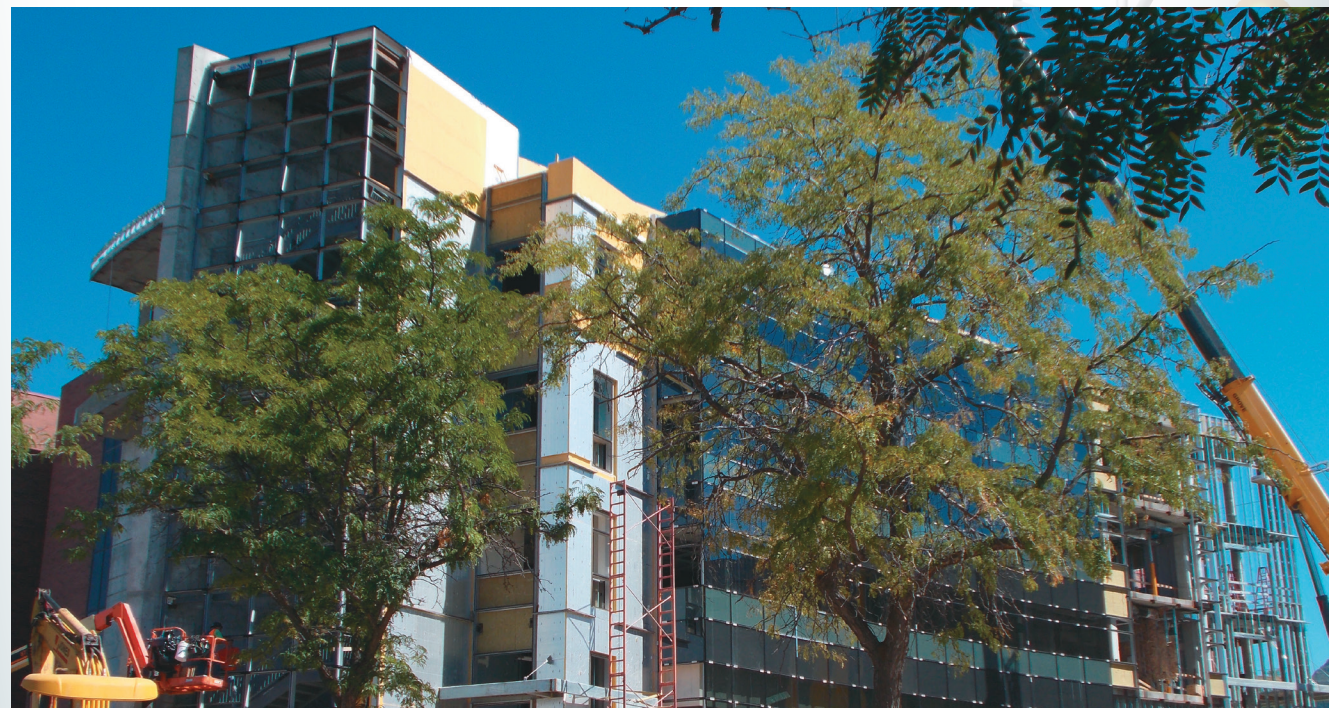
Southwest view of the new Thatcher Building for Biological and Biophysical Chemistry
